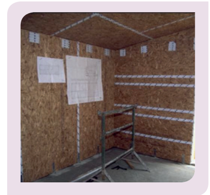
Figure 8 Specialist air tight adhesive tape is used to seal gaps between OSB boards
