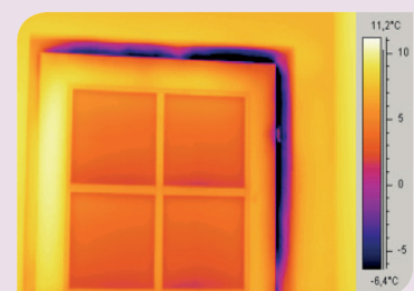
Figure 18 Infra-red thermographic image of air leakage between window casement and frame
